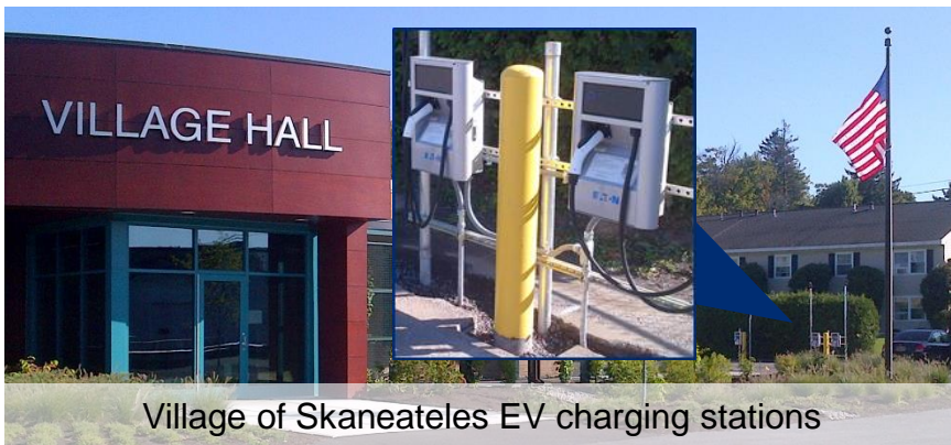
Town of Southold municipal EV charging
